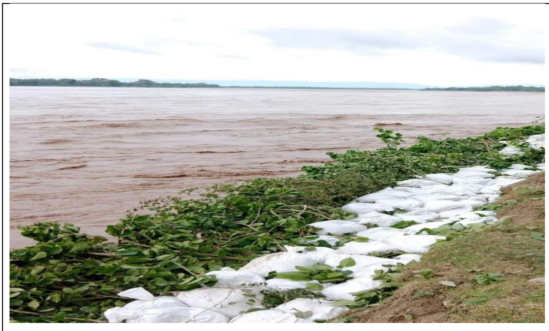
Figure 2: Wall in the bank of river made by using locally available resources(biodyke)
