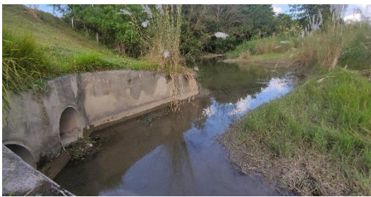
Water stagnation at AFS
