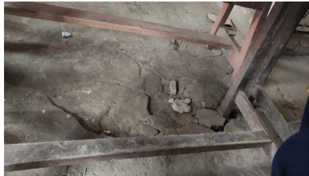
P. Damaged floor at classroom
