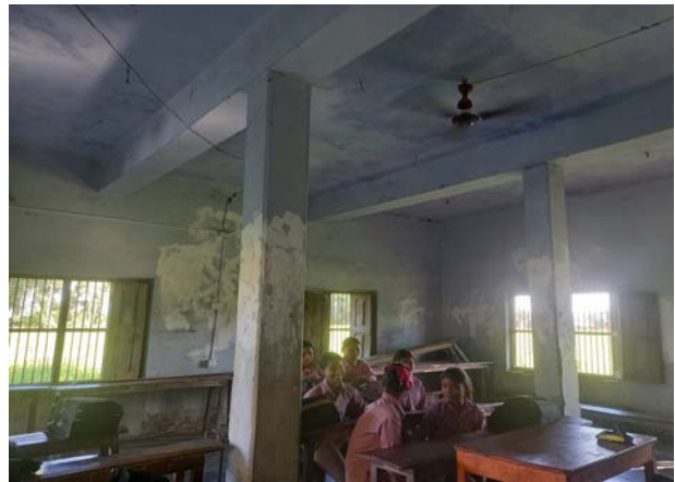
D. Students taking class in unrepaired classroom
