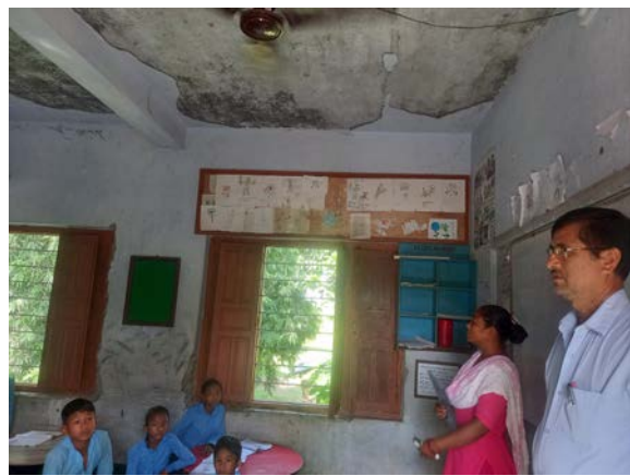
F. Students under damaged ceiling
