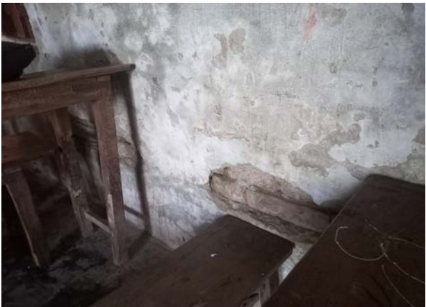
C. Damaged wall
